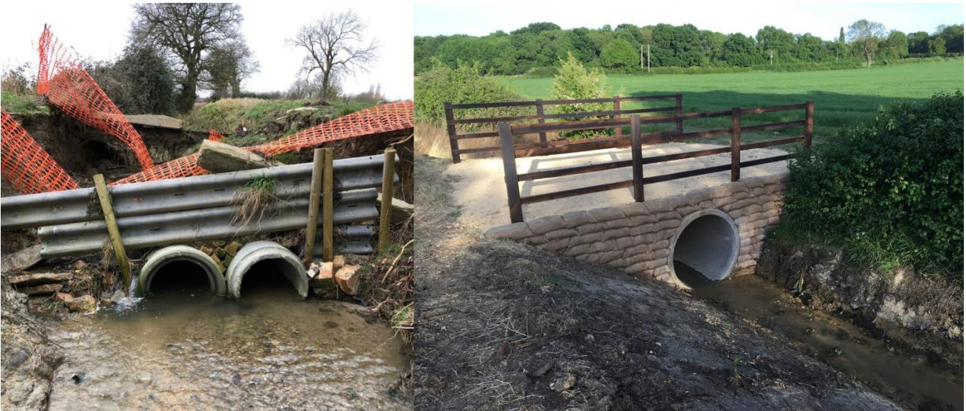
Figure 7-3 Culvert collapse and subsequent on Marholm Brook
